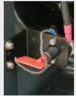
Battery cut-off switch
